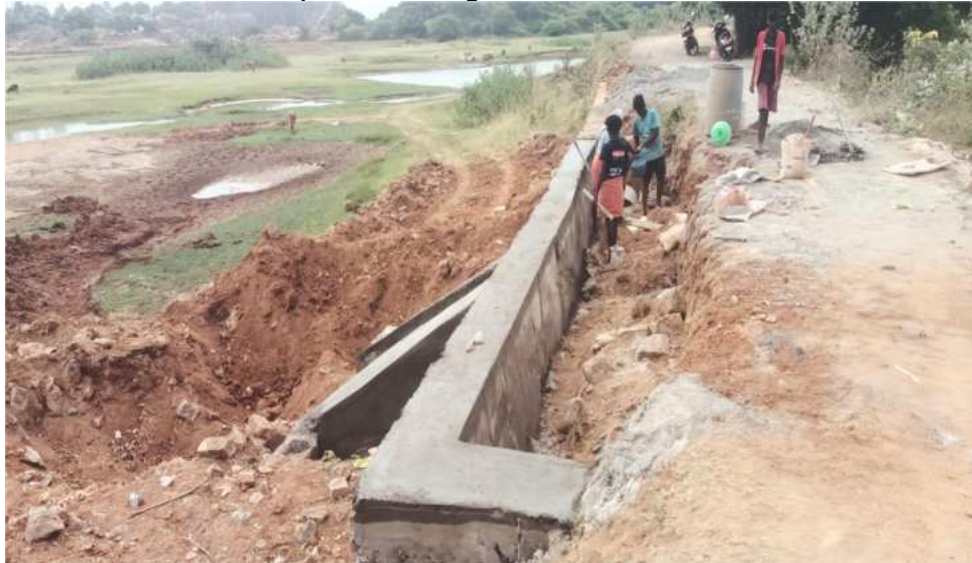
Permanent restoration of Tank bund erosion near Sluice No. 1 of Thuvrankulam in Pattapathu Village of Tenkasi Taluk in Tenkasi District
